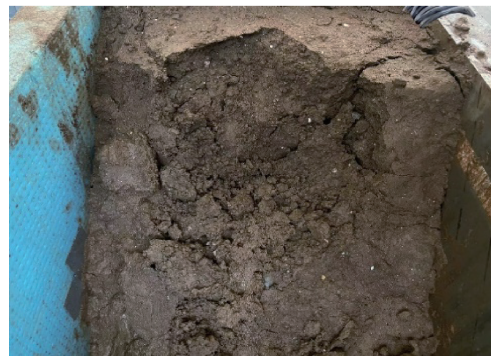
(c) 边坡崩塌破坏
